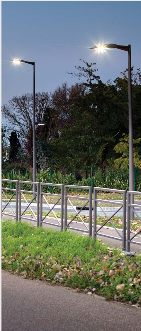
Selux Avanza- Roadway Poles
